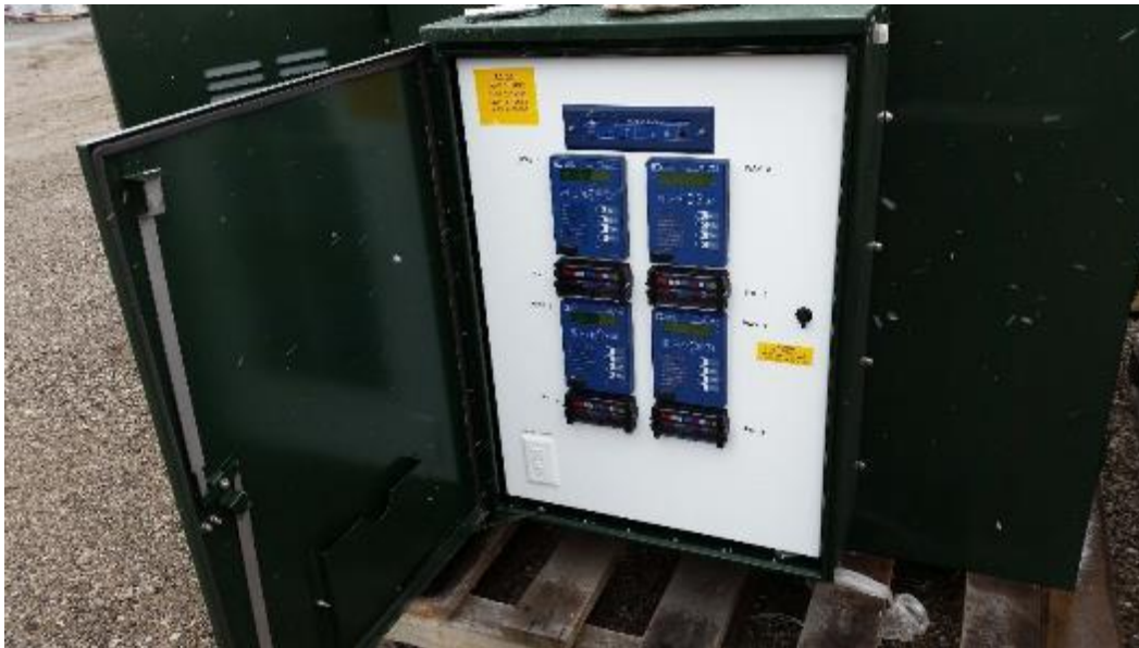
6 Figure A10 - 25: Automation Cabinet on Switchgear
