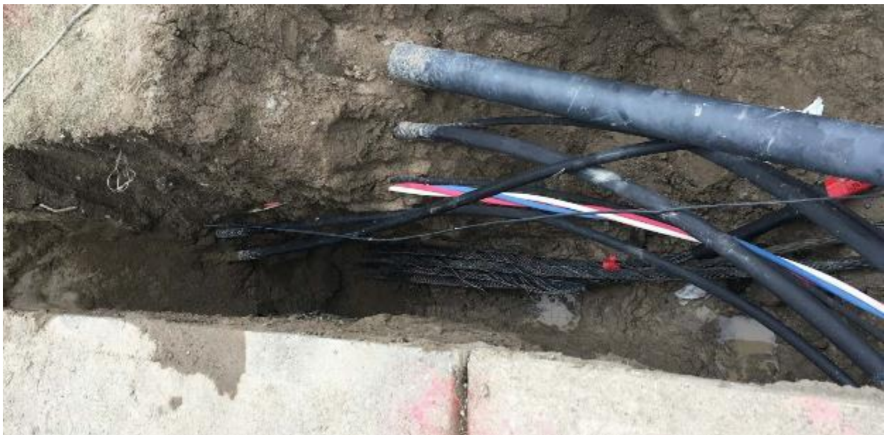
7 Figure A10 - 2: York Hilda Cable Trench
