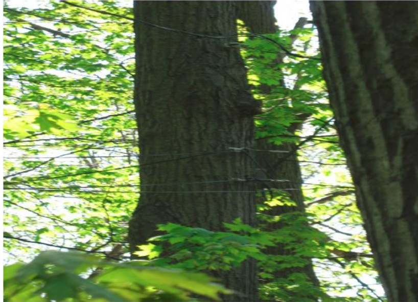
Figure A07 - 3: Secondary Distribution Conductor Attached to a Tree
