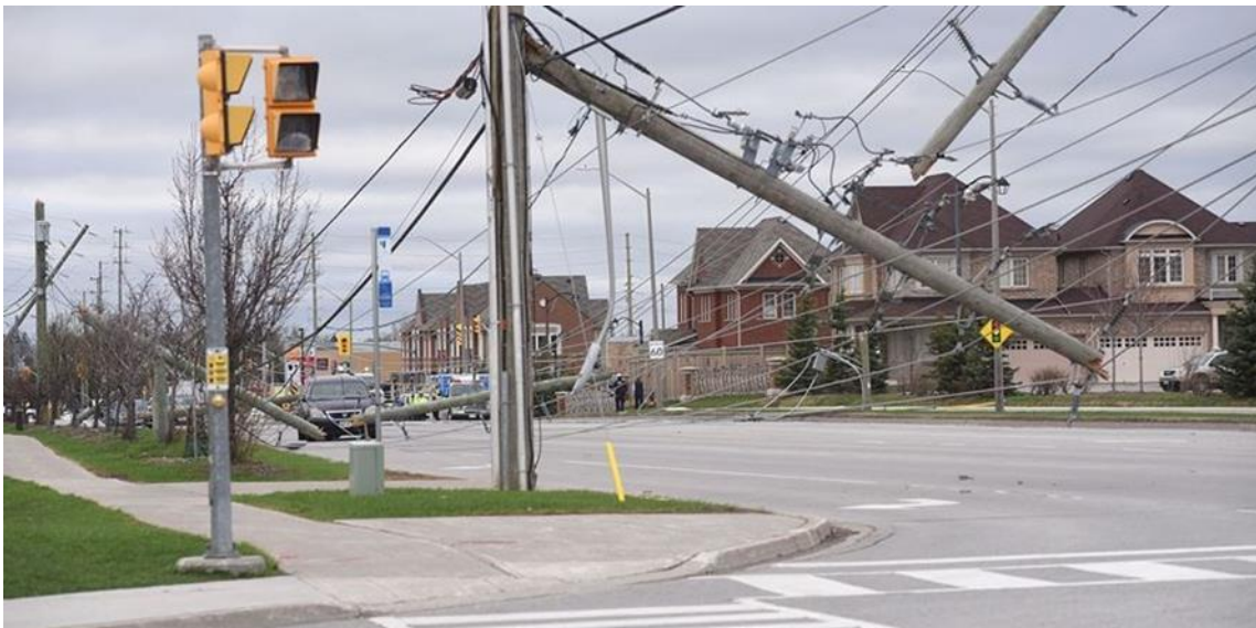
7 Figure 5.0 - 5: High winds caused downed power lines on Bayview Avenue in 2018
