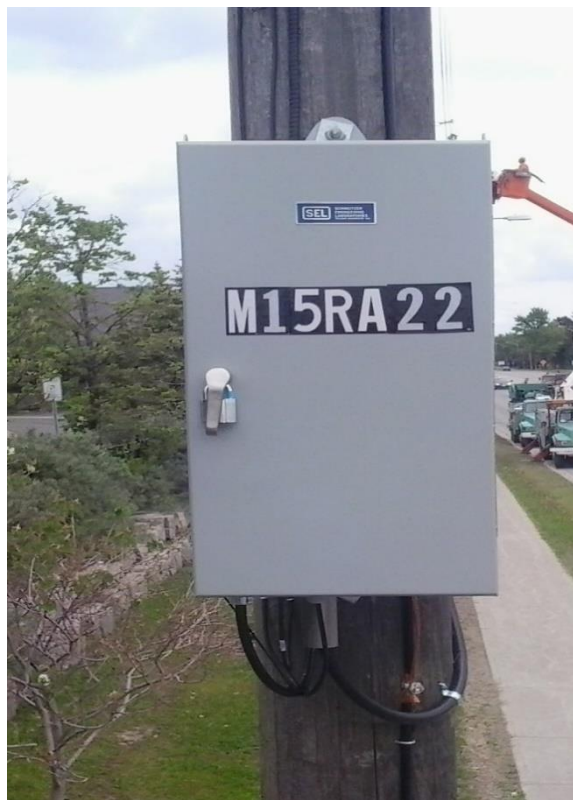
Figure A11 - 2: Control Box
