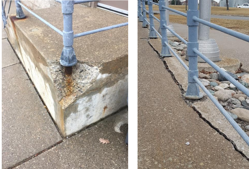
1 Figure A17 - 3: Water and Salt Damage of Wall at Sandalwood Parkway Building
