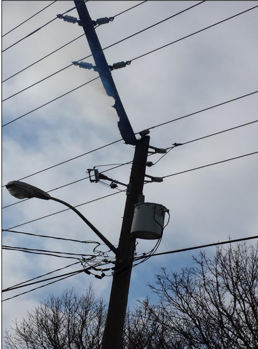
Figure 5.3.3 - 23: Pole Fire Event Alectra Utilities
