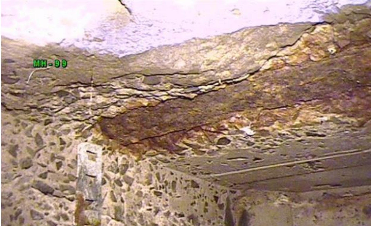
Figure A10 - 30: Lid Degradation: steel support rusting
