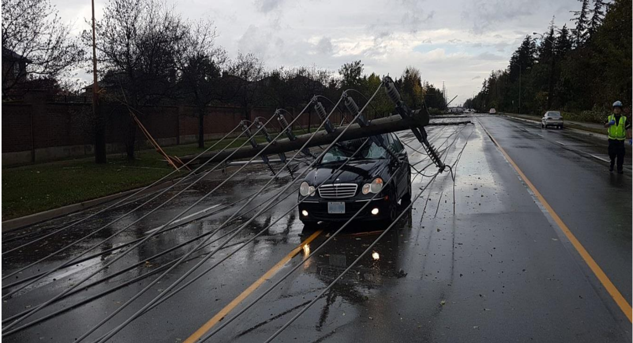
Figure A05 - 9: Failure of Legacy Wood Pole on October 15th, 2017
