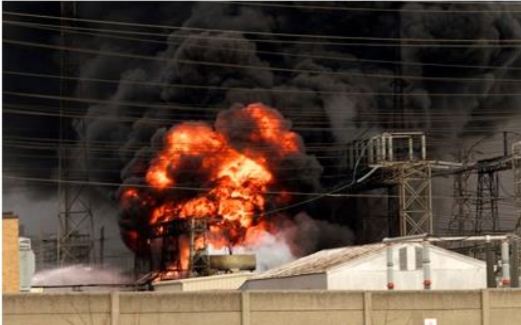
1 Figure A08 - 1: Explosive Failure of a Hydro One Transformer at Richview TS on March 18, 2011
