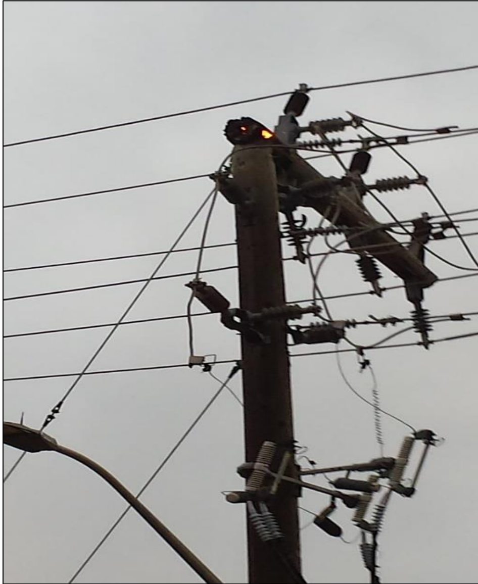
Figure 5.3.3 - 22: Active Pole Fire Event Alectra Utilities
