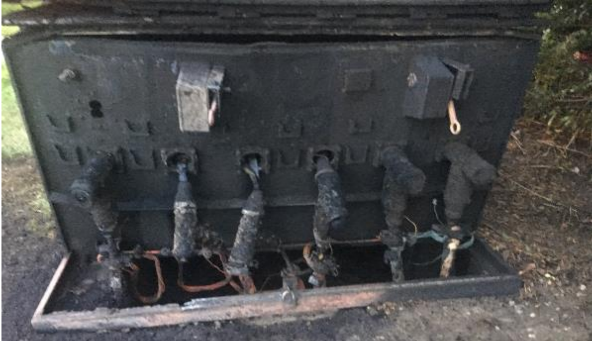
Figure A10 - 22: Failed Oil Filled Padmounted Switchgear
