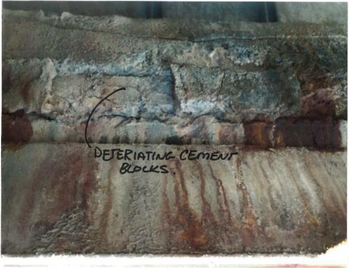
Figure A10 - 31: Lid Degradation: Cement crumbling
