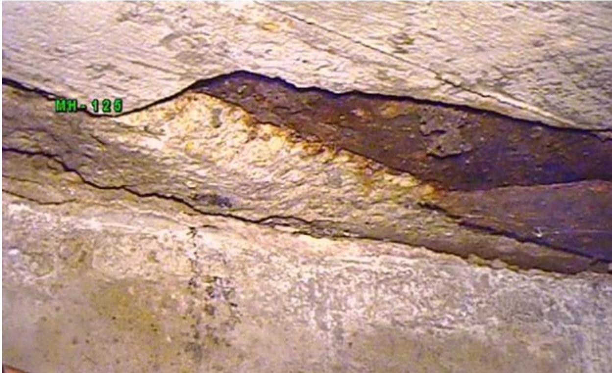
4 Figure A10 - 29: Lid Degradation: steel supporting rusting
