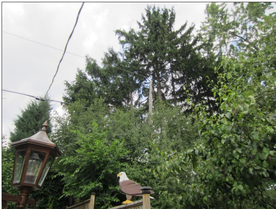
14 Figure A07 - 2: Inaccessible Pole in Poor Condition (cracked and rotten)
