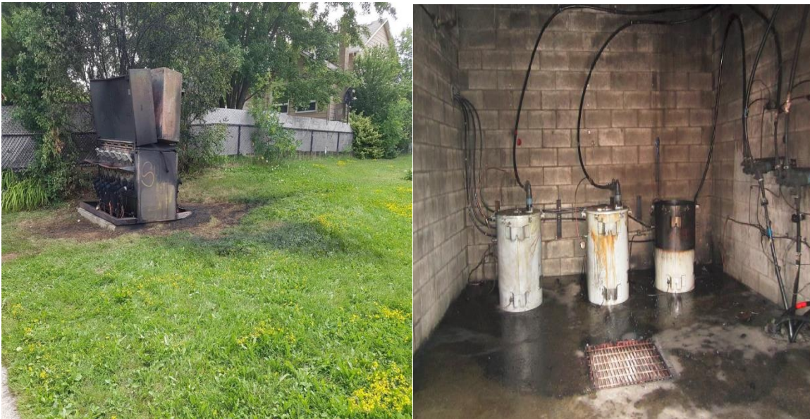
13 Figure A06 - 1: Catastrophic Failure of Switchgear and Vault Transformer
