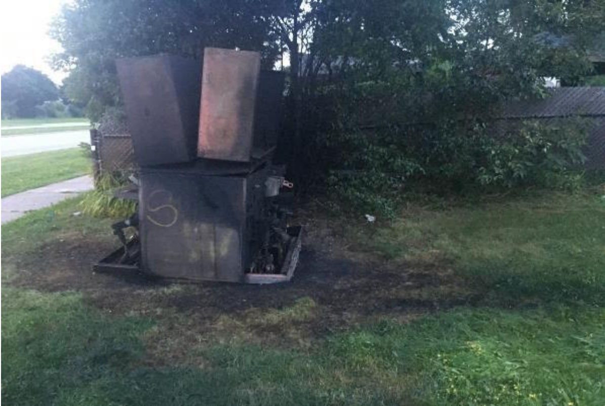
Figure A10 - 15: Failed Oil-Filled Switchgear, August 2018
